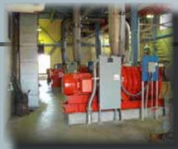
Forward Flow Aeration System
