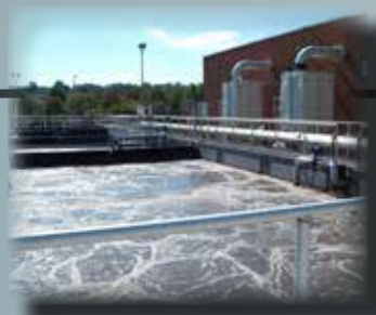
Aeration/Anoxic Post-Aeration Zones
