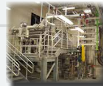
Biosolids Drying Facility Indirect Dryer System
