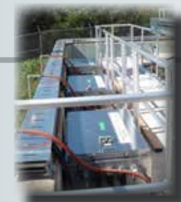
UV Disinfection Facility
