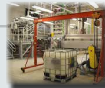
Biosolids Drying Facility Centrifuge
